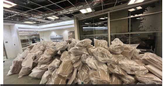
Interior photos of City Hall during remediation and construction following June fire and water damage.
